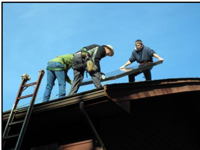
Nothing but blue sky and sunshine on this beautiful October day for one of our many Neighbors-helping-Neighbors solar hot water installations. Safety is always first with the Roof Team wearing harnesses as they put a solar collector into position.
